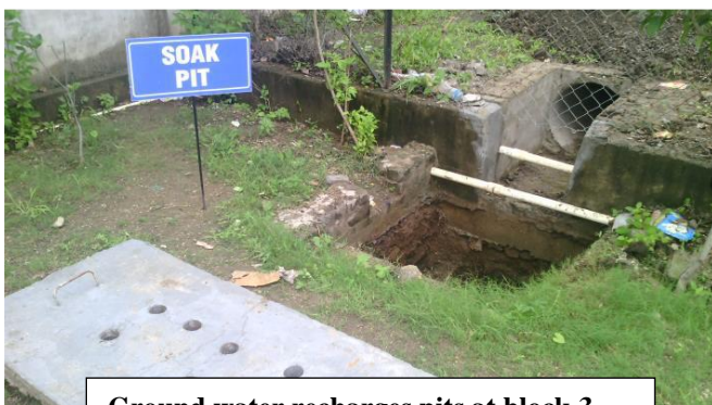
Ground water recharges pits at block 3
